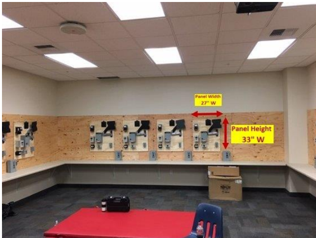
MOTOR ROOM – panels (example only)
